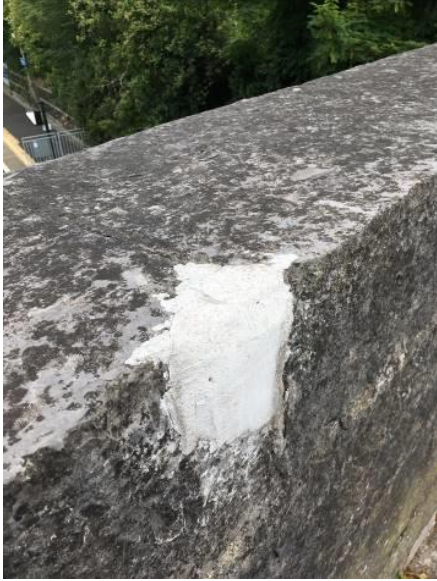
Figure 22 – Poor mortar repairs to copings.
