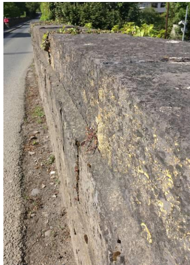
Figure 25 – Coping does not extend to internal face of wall.
