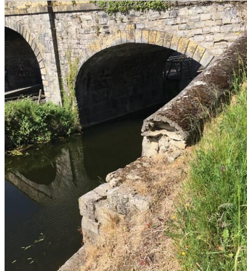
Figure 23 – Top of pier lost, exposing end of modern concrete copings on north west wing.
