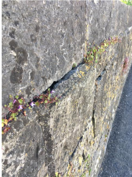
Figure 33 – Stonework and pointing on parapet to be repaired.
