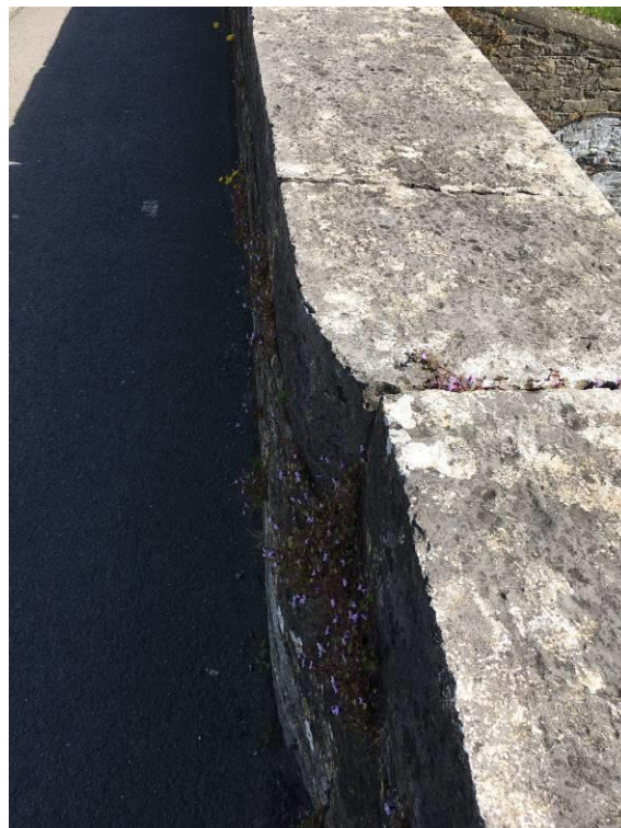
Figure 14 – View taken looking down on coping stones on Cope Bridge's north east parapet, showing the depth of the wall top extending into the bridge.
