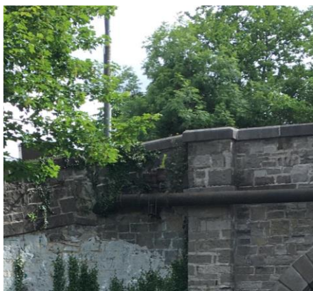
Figure 16 – Poorly rebuilt stonework around service pipe on north west side.
