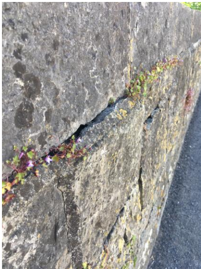
Figure 24 – Mortar broken away from coping stone.
