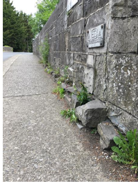
Figure 23 – Stonework at base of wall requiring pointing.
