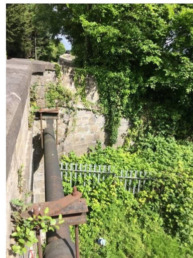
Figure 6 – North east wing wall with substantial block repairs.
