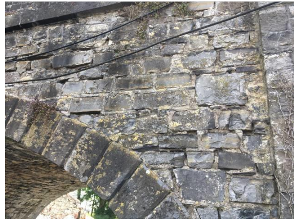
Figure 19 – Pointing loss on spandrel.
