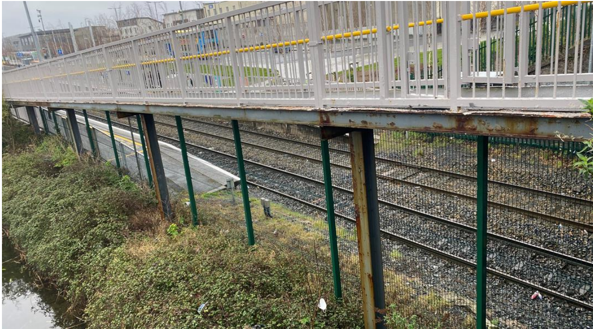
Figure 3-5 Steel corrosion on beams and supports
