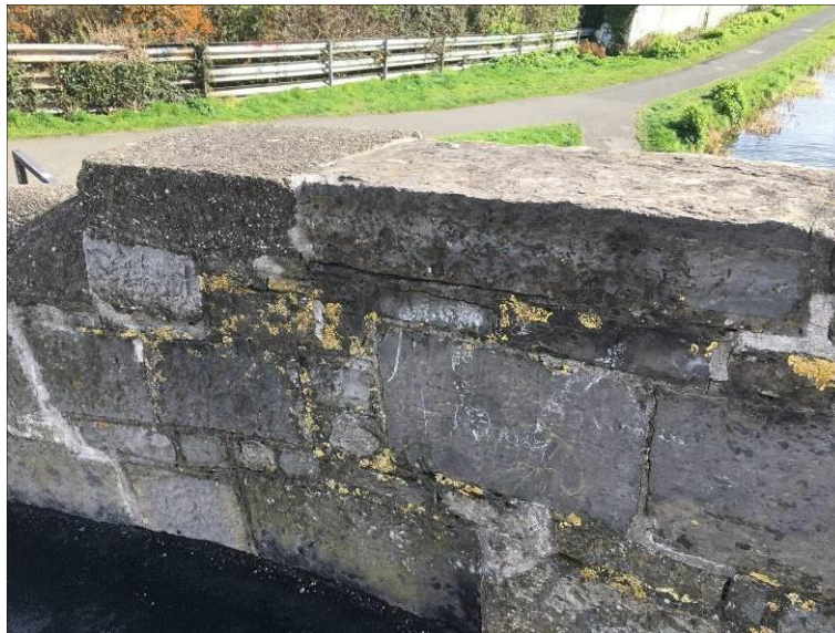
Figure 30 – Existing parapet requires repair and conservation works.
