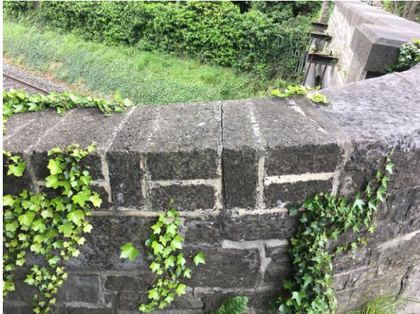
Figure 18 – North east parapet repaired in blockwork with cracks visible.
