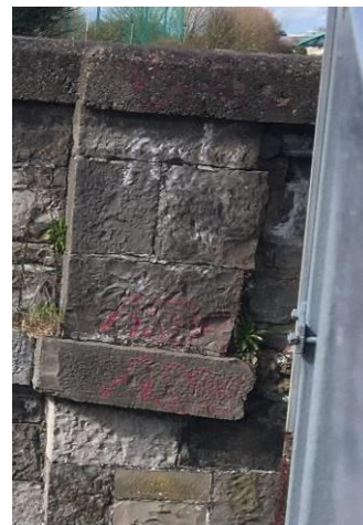
Figure 24 – Pier stone damaged.
