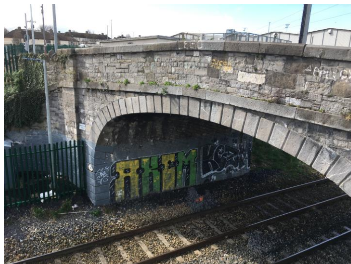
Figure 20 – Graffiti under railway arch.
