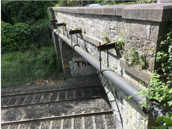
Figure 14 – Painting and graffiti under the bridge.
