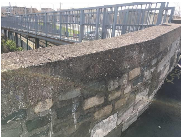
Figure 23 – Poor condition of pointing & concrete copings.
