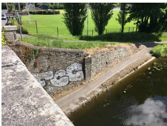
Figure 20 – North West canal wing wall.
