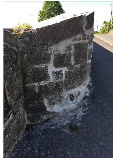
Figure 26 – Recent repairs to north east corner.
