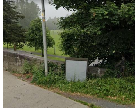
Figure 8 – North west parapet.
