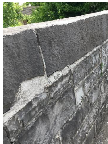
Figure 21 – Joint below coping stones broken.
