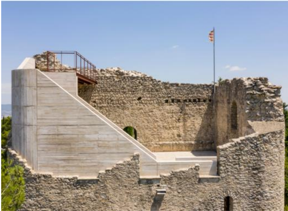
Figure 26 - Example of a new board marked concrete insertion in an existing stone structure.
