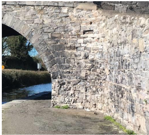
Figure 18 – Weathered facing stone visible, especially below the spring of the arch.
