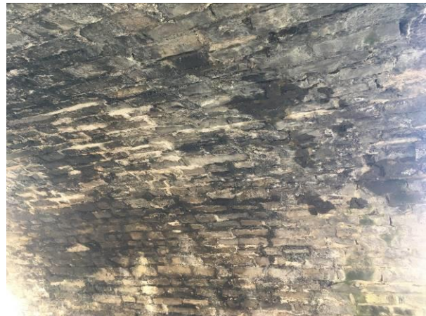
Figure 19 – Condition of canal arch stonework.
