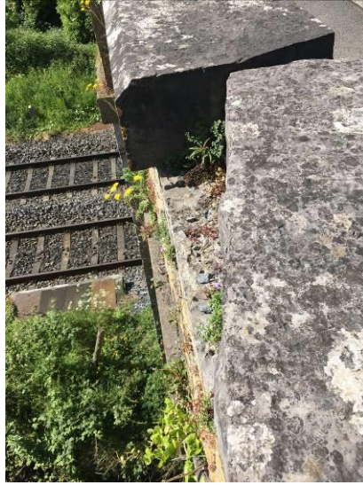
Figure 27 – Lost section of coping stone over canal.
