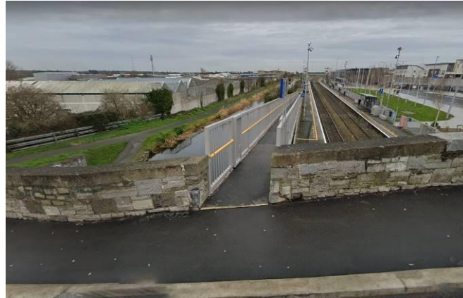
Figure 5 – Breach in east parapet wall.
