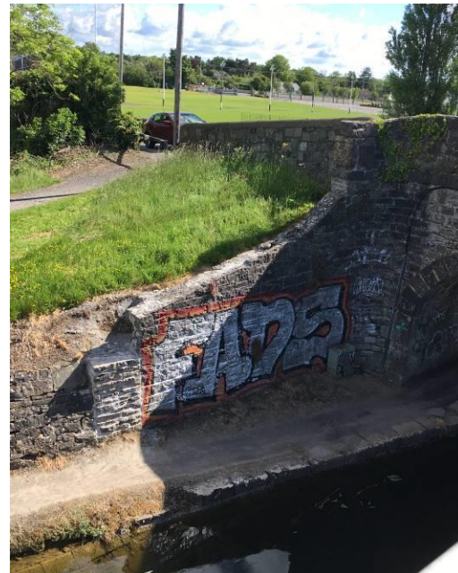
Figure 5 – North west wing wall with pier recently rebuilt. Note the wall is missing coping stones...
