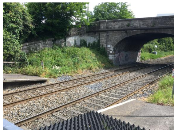
Figure 17 – Vegetation and paint on north west wing wall and paint under bridge.
